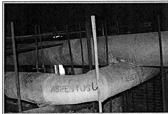
Asbestos in Building #23
