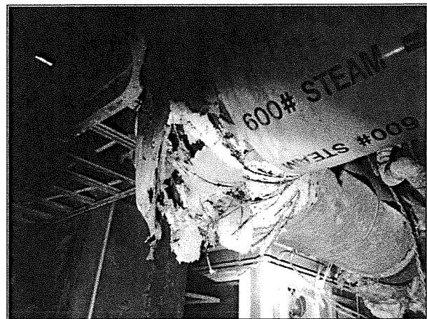
Building #23 Interior asbestos material
