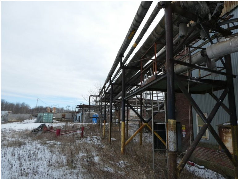
Powerhouse Building 23 Pipe Rack West Side
